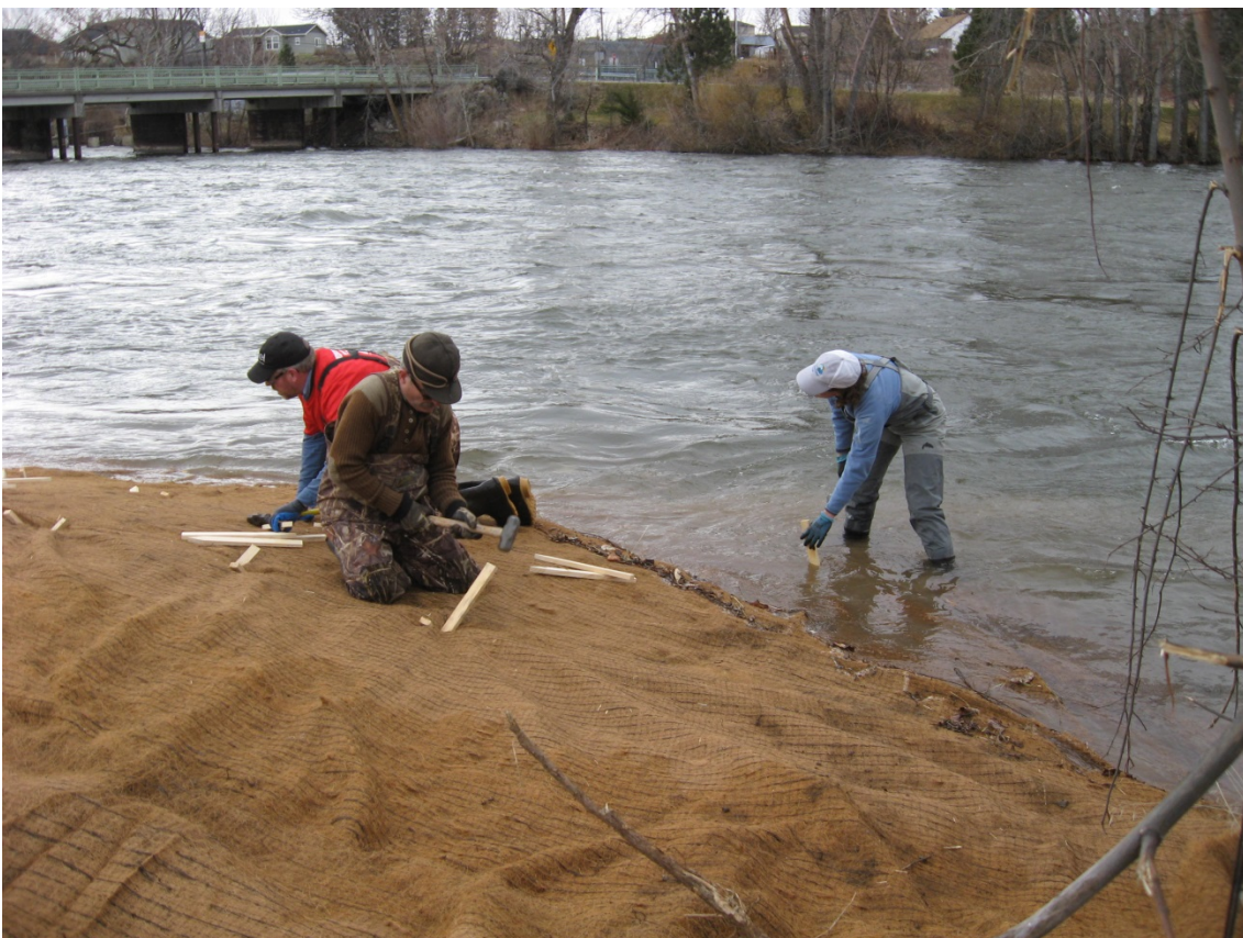
January 22, 2017 - Background shows water completely covering engineered log jam on south bank
