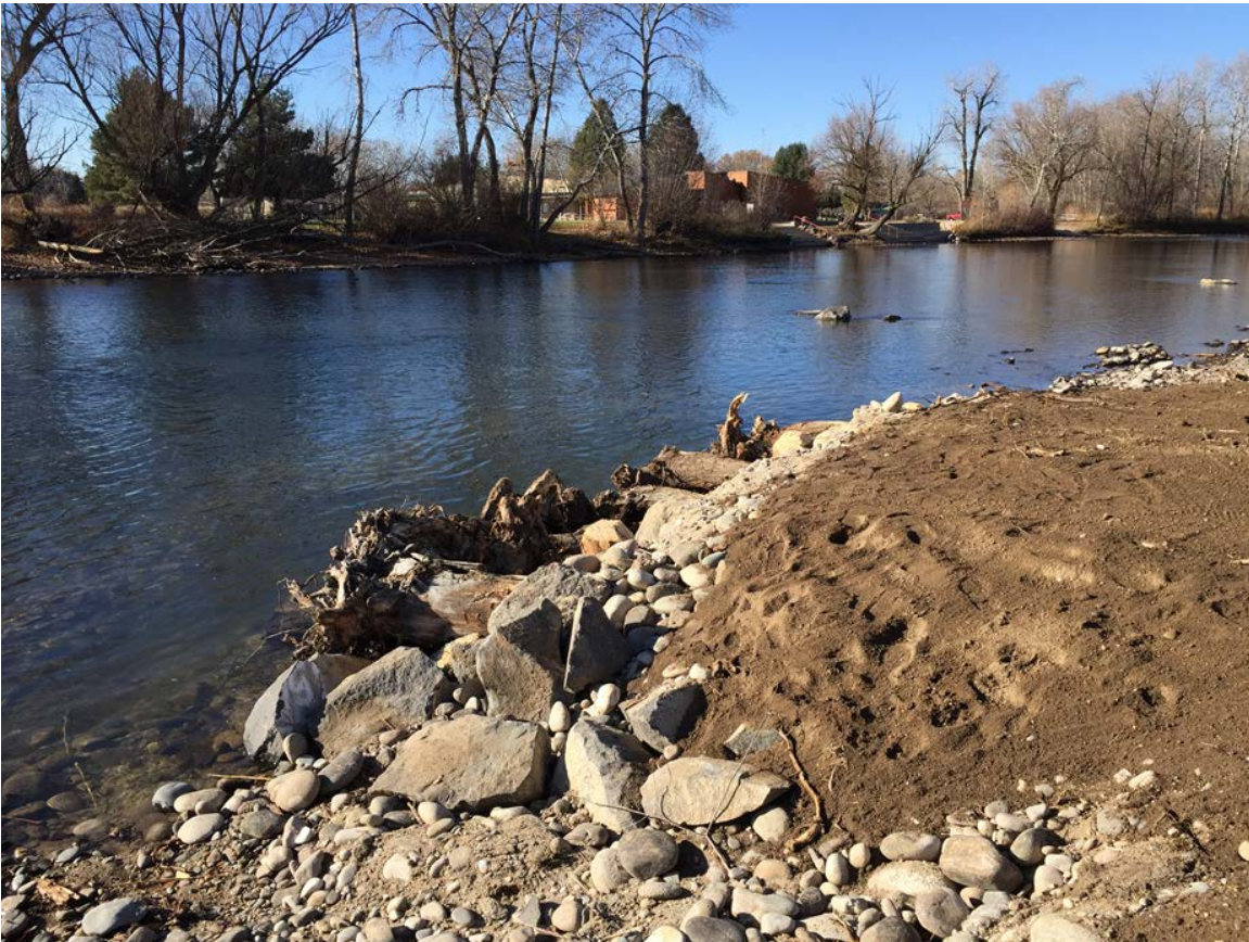
December 9, 2016 - Engineered Log Jam showing top soil area to be planted in early 2017
