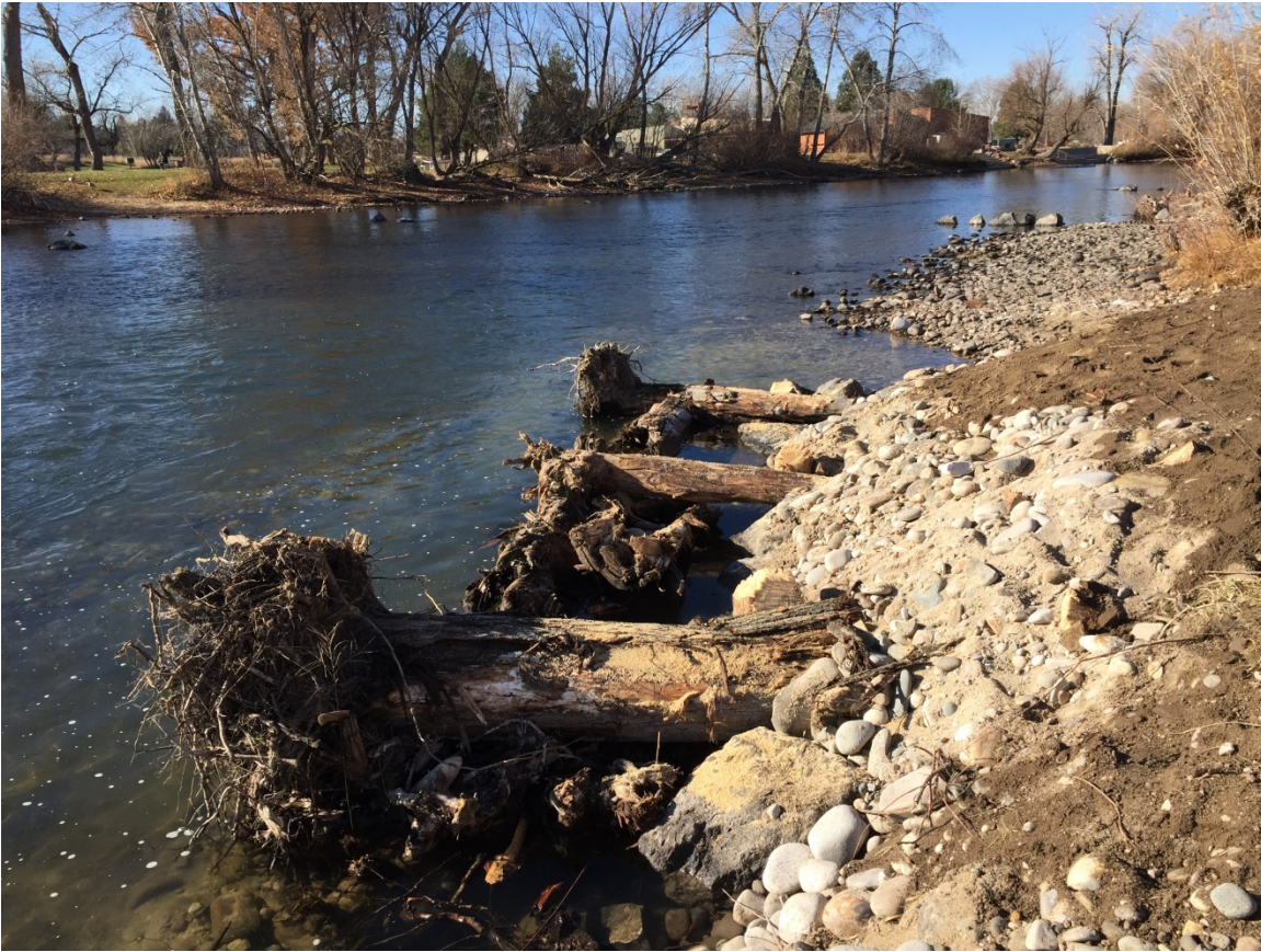
December 9, 2016 - Engineered Log Jams installed on north side of Boise River, across from Barber Park
