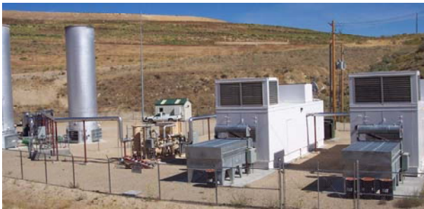
Electricity co-generation facility.
