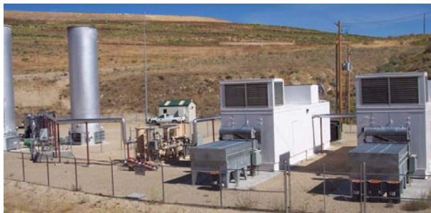
Generator sets (white containers on right).
