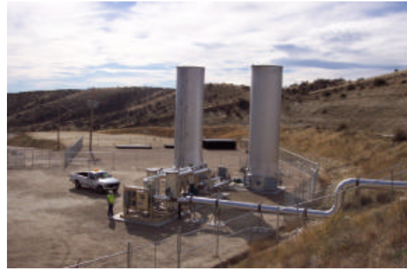
Figure 11 LF Gas Flare Station
