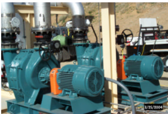
Figure 10 Motors and Compressors
