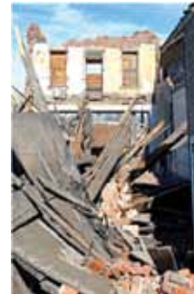
Moderate earthquakes can cause devastating damage to older masonry buildings. This photo shows a roof fall that occurred during the 2008 M 6.0 earthquake in Wells, Nevada. Earthquakes of this magnitude can occur anywhere in Idaho. (NBMG photo.)
