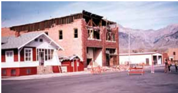
Earthquake damage to the Custer Hotel in Mackay, Idaho caused by the 1983 M 6.9 Borah Peak earthquake. (IGS photo)
