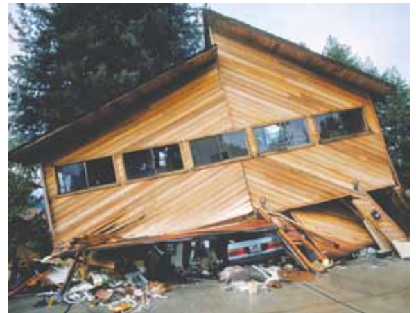
This home in the Santa Cruz Mountains collapsed in the Loma Prieta earthquake. (Photo courtesy of USGS)
