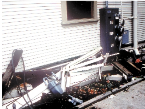
Cripple wall foundation failure and utility damage, Northridge, Calif.
