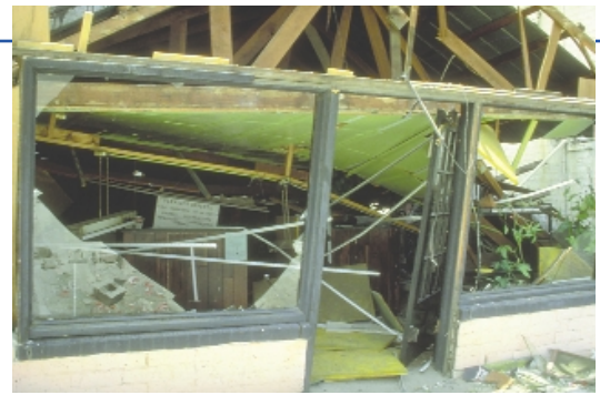
Damaged building, Coalinga, Calif.
