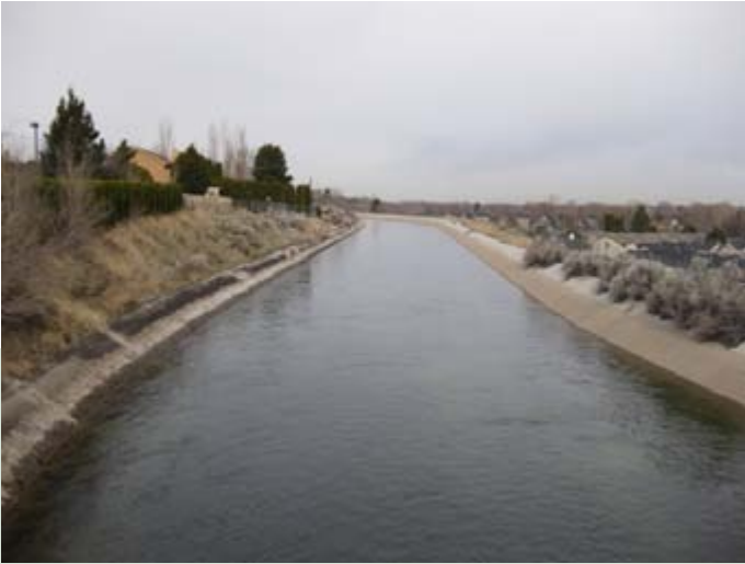
Figure 31: New York Canal Boise, Idaho
