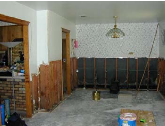
Figure 35: Flood damaged home.
