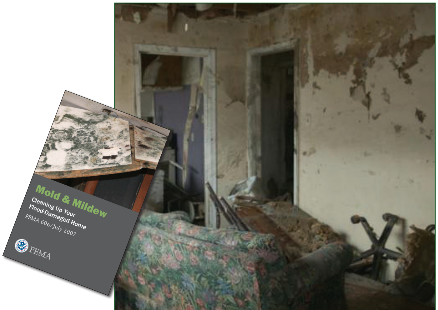
Figure 36: Flood damaged home..
