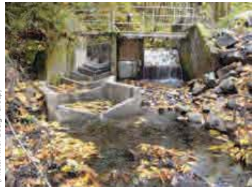
Rock Creek, OR. A fish ladder was constructed to provide fish passage around an irrigation structure.
